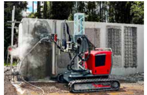
Aquajet showed its fleet of equipment and performed hydrodemolition demonstrations at the company's 2024 World Tour event in Germany.
