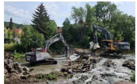
A second, smaller excavator plus hammer and bucket, broke out the individual concrete segments, and transported them to the riverbank.
