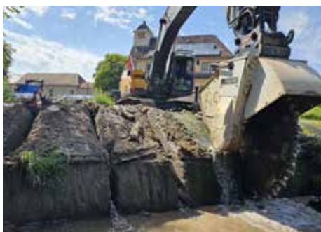
Using a KEMROC cutter wheel on a 32t excavator, the massive concrete weir wall was cut into individual segments.
