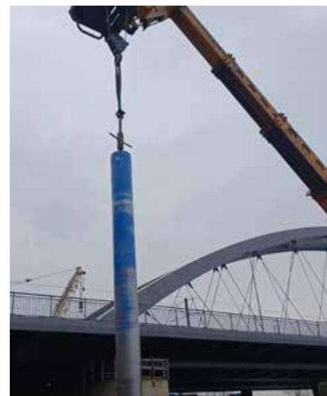
The already assembled screw drill bits were moved to the right places by crane.
