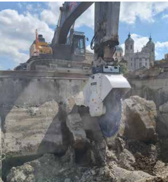
Massive concrete structures have to be demolished before a new multi-purpose quarter can be built.
