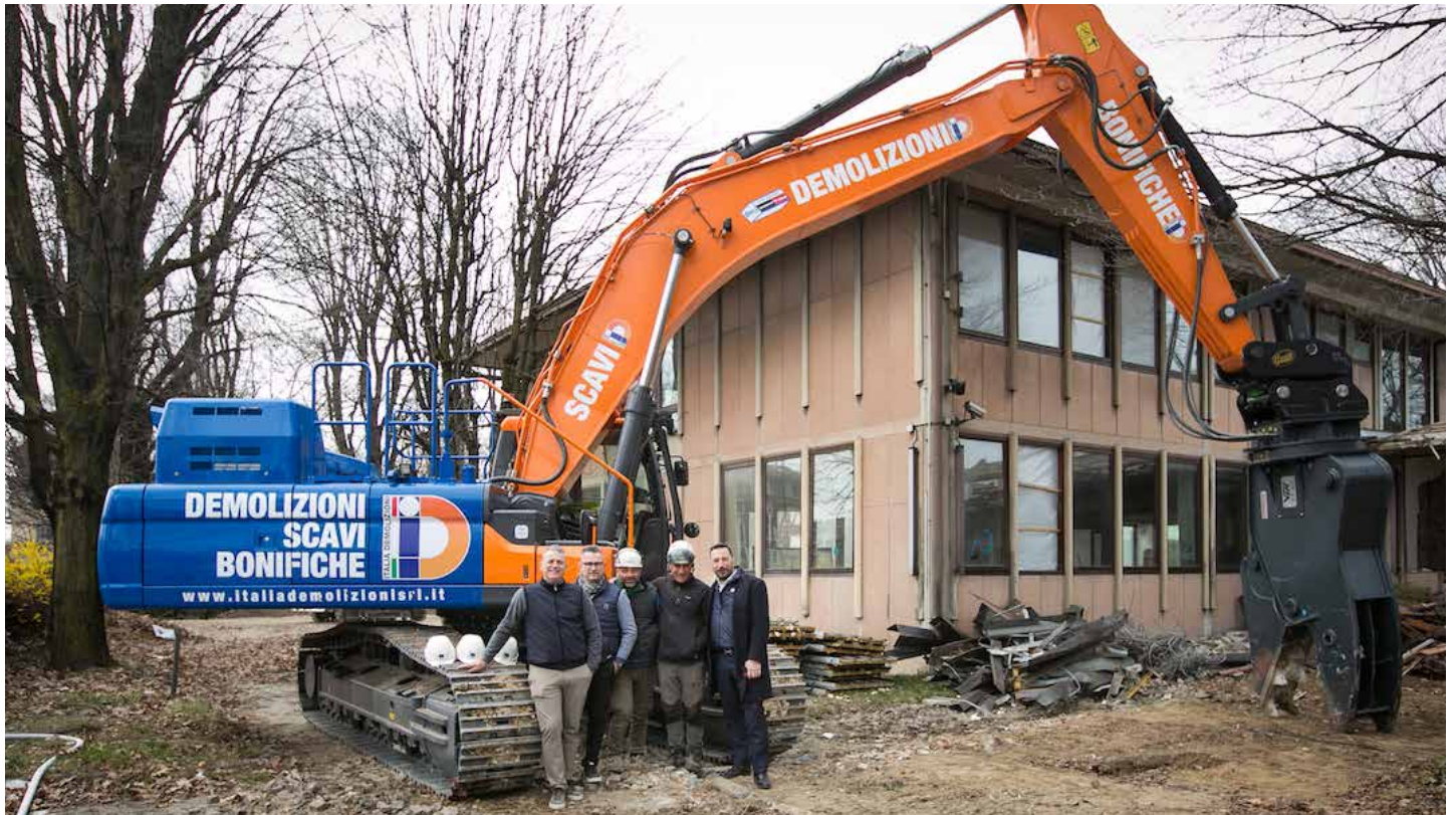
From left, Nicola Miceli, owner of A.C.M. and Italia Demolizioni; Ivano Perego, commercial director of Italia Demolizioni; Alessandro Migale, site technical manager of Italia Demolizioni; Ernesto Perego, demolition operator and Pier Francesco Marcotto, Italy Demolition Division manager.
