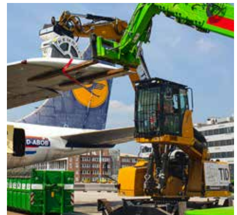
The end of a veteran has arrived: On June 10 th 2021, demolition experts from TID scrapped a 65 year-old Boeing 707. They used a KEMROC KDS 50 diamond saw mounted on their telehandler.
