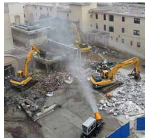
Surrounded by buildings on all sides, the concrete buildings are carefully broken down by excavators.
