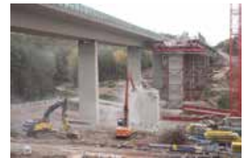
Wende is using heavy duty machine technology to demolish the motorway viaduct at Langenschwarz, including using three excavators fitted with Genesis demolition shears.
