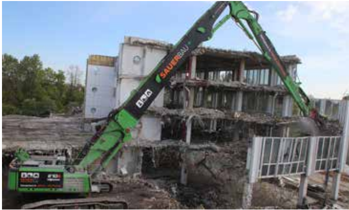
The 870 E long front demolition material handler carrying out controlled demolition in crowded downtown Munich.
