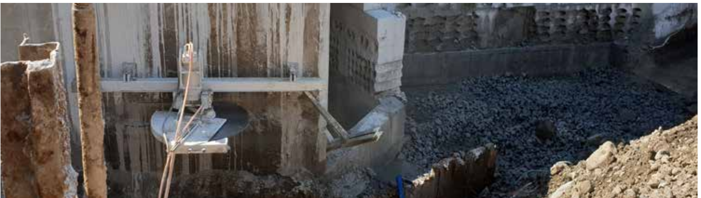
Below a Pentrunder wall saw cutting at the large infrastructural project “Slussen” in the center of Stockholm.
