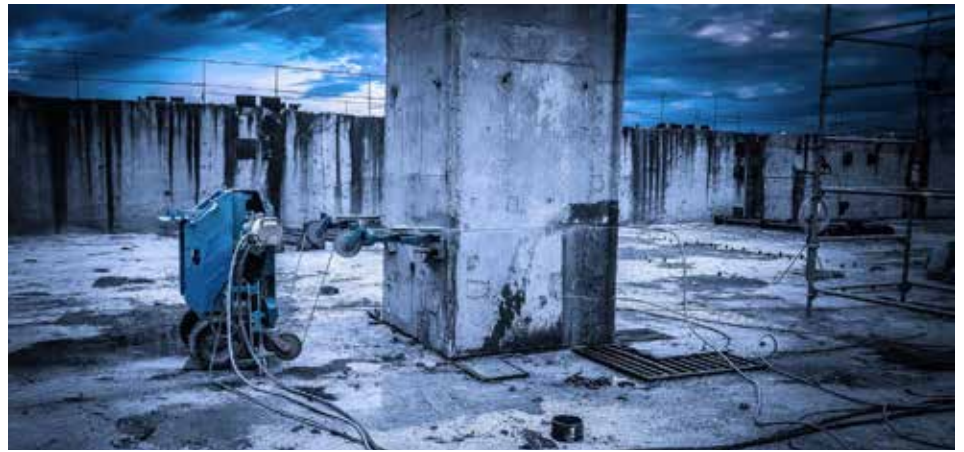
Cutting of a reinforced concrete column with the wire saw SB-E. (Photo: Diamond Drilling)
