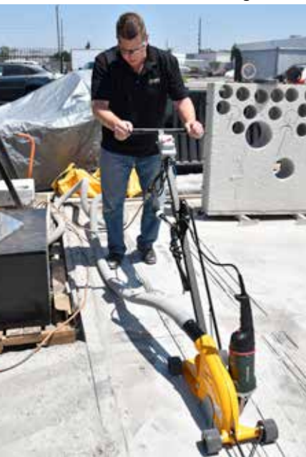
Dave Glynn operating a "dust buggy". It's a kind of joint cleanout saw that cleans out joints and collects dust and debris at the same time;
