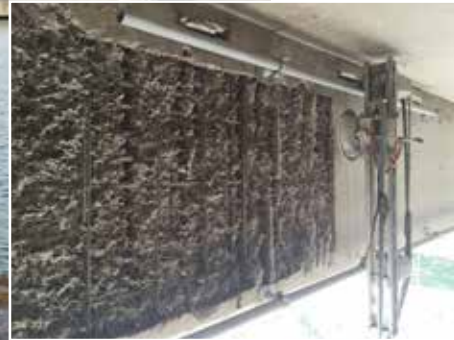
Picture to the left: The Nalta 101 installed under the quay along one of the crossbeams.
