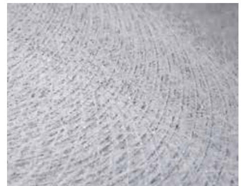
The profile has been endorsed by topping and resin manufactures to give a proper CSP3 bonding surface with their products.
