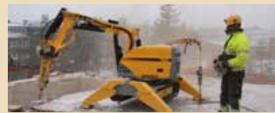
Greasing before and during operation also is part of proper breaker maintenance that reduces equipment wear.
