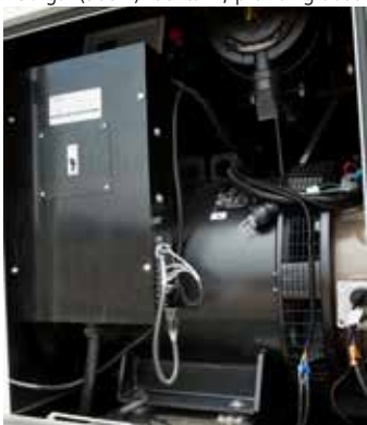
The unit is powered by a 480V/150kW generator with a 6.8 L John Deere Tier III flex diesel engine.
