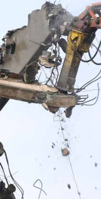
Silverado Contractors' high-reach excavator and Atlas Copco's HB 2500 breaker knock out Candlestick Park's concrete wind baffle.
