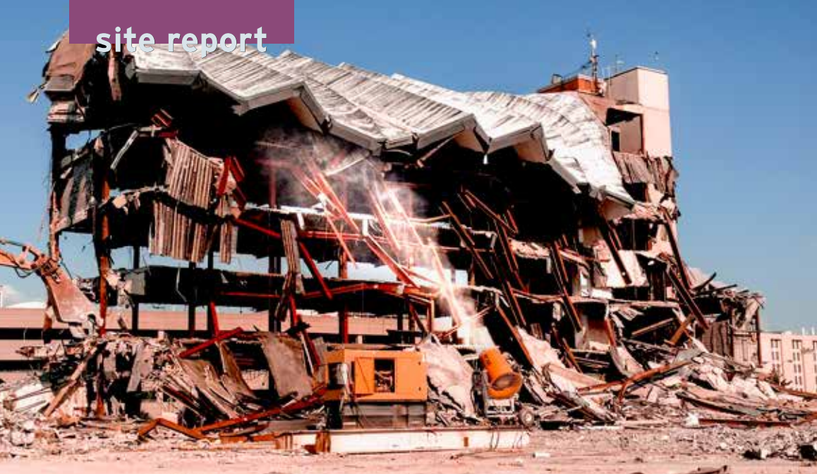
To effectively control multiple dust-generating sites, Veit built a skid and mounted the DustBoss with a diesel-powered generator.
