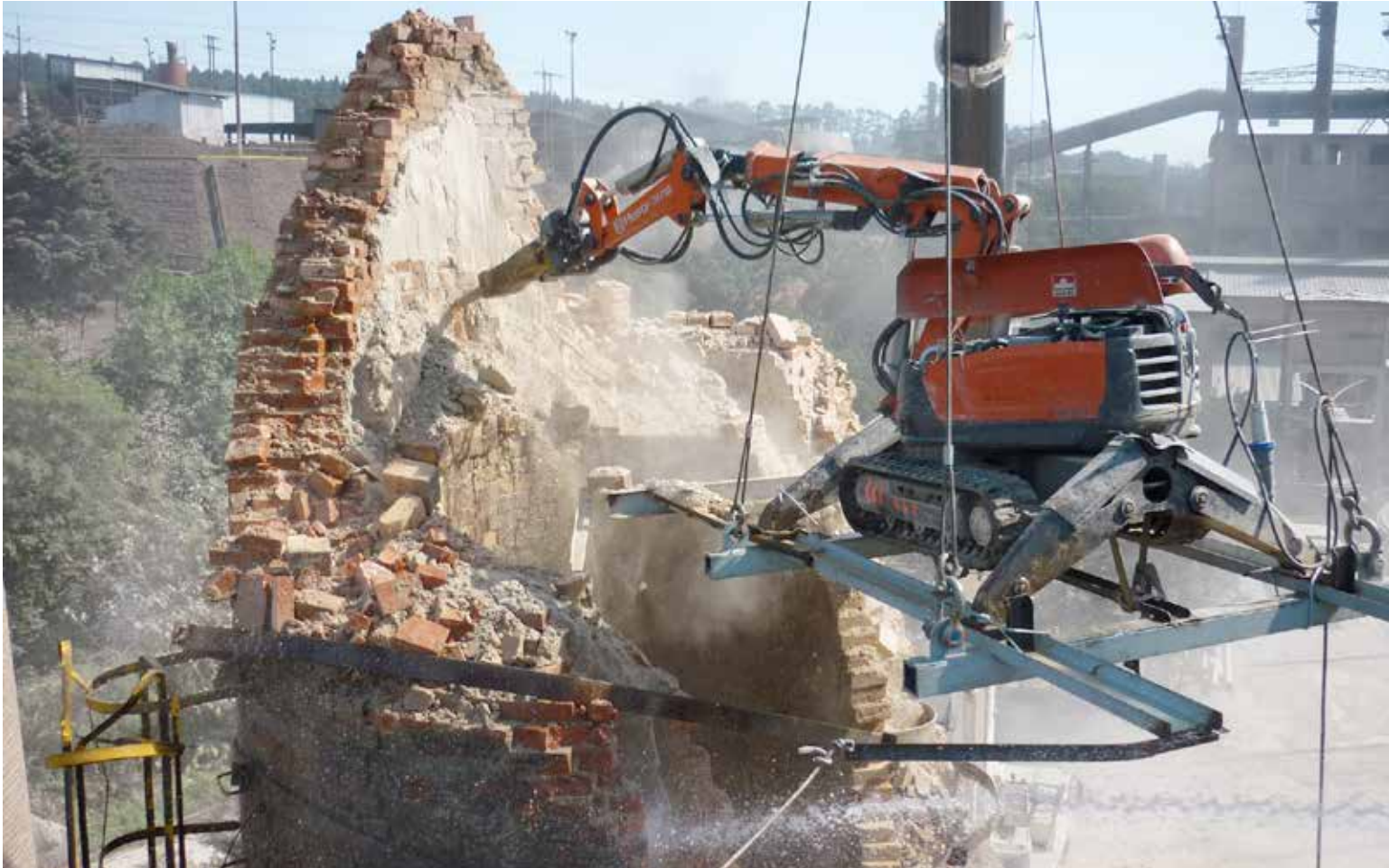
Knocking down a 45 m chimney in the Brazilian state of Para with a remote controlled demolition robot from Husqvarna.
