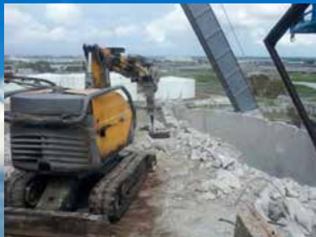
The compact Brokk 180 was light enough to sit on the roof of the structures yet powerful enough to break up the tough concrete.
