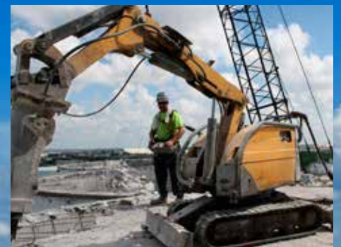
The remote-controlled Brokk allowed the operator to remain a safe distance from the work, while maintaining a clear view of the demolition.
