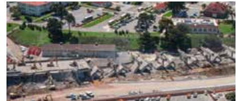
The Presidio remained open to the public during demolition, so the contract called for a control plan to prevent dust from leaving the project boundaries.
