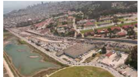
Demolition of the old structure involved approx. 4,700ft (1.4km) of roadway, including 150 spans, yet the plan allowed complete road closure for just one weekend.
