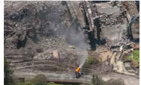
One full-oscillation DB-60 can cover nearly 125,000ft 2 (more than 11,600m 2 ) with a highly efficient dust-trapping mist.
